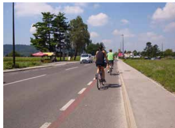
The reconstruction of the road Litijska cesta was carried out within the European project Clean for You, with which we are expanding the sewage system, and in parallel with the renewal of the road surface, we are making sure the traffic regulation is appropriate, thus ensuring greater traffic safety. Photo: Kristina Ina Novak
