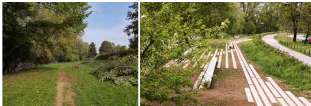
BEFORE The left bank of the Ljubljanica River before the renovation. NOW In parallel with the refurbishment of the brownfield site, we have also renovated a part of the left bank of the Ljubljanica River, where we created a new public space with a walking path, benches and sunbathing surfaces for spending free time (Muste beach). Photo: Helena Regina
