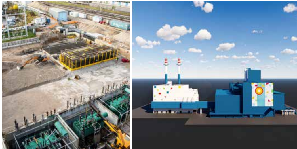
We are looking forward to the completion of the gas and steam unit in the existing heat and power station TE-TOL, with which we are going to reduce the use of coal and ensure even cleaner air in Ljubljana. Photo: Urban Štebljaj and archive of Energetika Ljubljana
