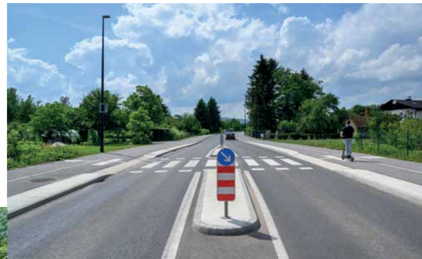
One of the most important improvements to the road and municipal infrastructure within the Clean for You project is the comprehensive renovation of the Cesta dveh cesarjev from Cesta V Mestni Log to Barjanska cesta, which includes a new roundabout. On both sides of the road, we arranged a sidewalk and a bicycle lane, and for greater traffic safety, we also implemented several traffic calming measures with speed bumps, centred islands, and stationary speed meters.
