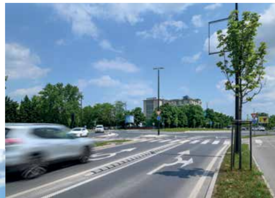
In 2022, as part of the renovation of Letališka cesta, we arranged new bicycle and pedestrian paths. In 2021, the reconstruction of the Letališka cesta connection to the Ljubljana ring road (DARS) was also carried out, and a bridge for pedestrians and cyclists over the ring road was also built.
