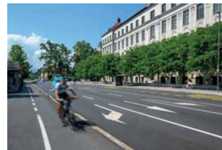
On Barjanska cesta, by reconstructing the section of road from the intersection of Gradaška ulica and Finžgarjeva ulica to the intersection with Slovenska cesta, we arranged the missing bicycle surfaces, provided more space, and established better-quality surfaces for cyclists, separated from pedestrians.
