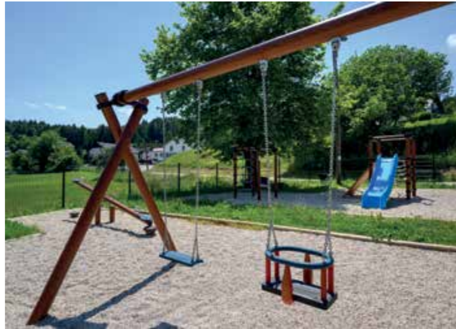
We renovated the children's playground in Stanežiče as part of the small works project.
